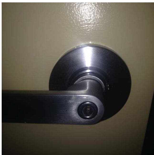
Photo 6. Lock on pre-school washroom.
