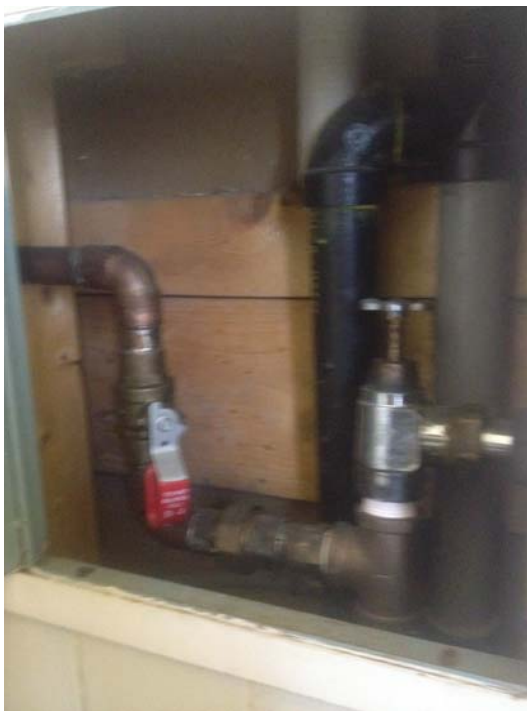
Photo 20. Valves located in cabinet above rink-side washroom toilet.
