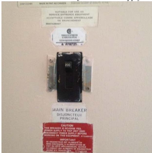
Photo 16. Main breaker for electrical supply.
