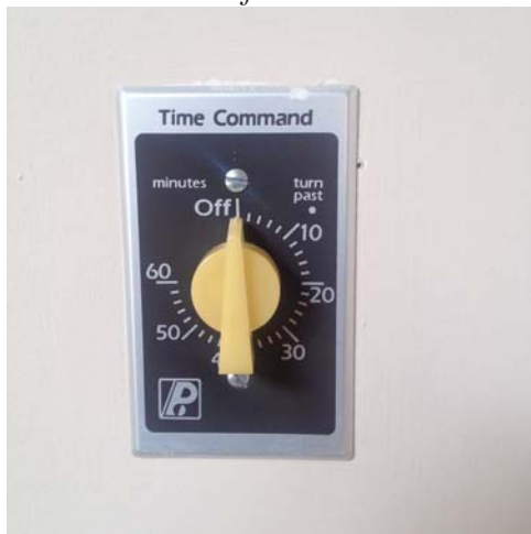
Photo 14. Timer for main hall ventilation
