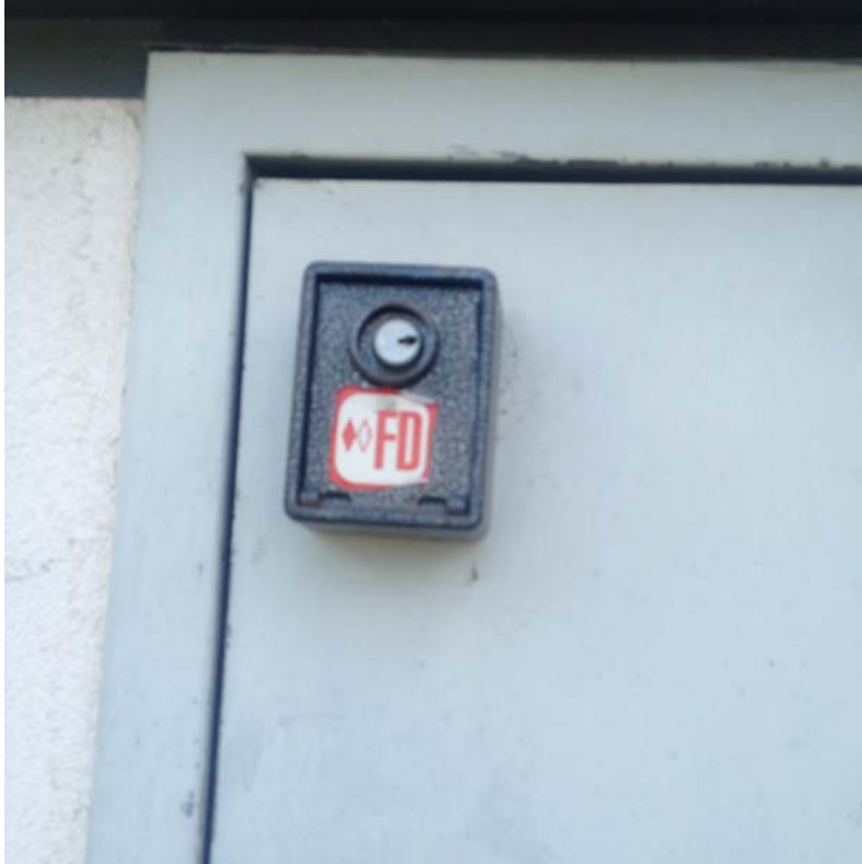
Photo 11. Key box for Fire Department to access master key.
